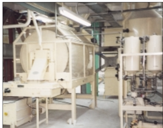
Continuous mixing plant in the Dominican Republic
